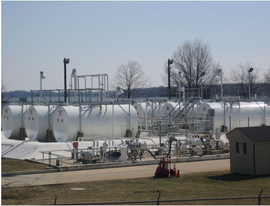
12,000-Gallon Aviation Gasoline (FF-1A and FF-2A) and Jet A Fuel Tanks (FF-3A, FF-5A, FF-6A, and FF-7A) At Fuel Farm – East Containment Area
