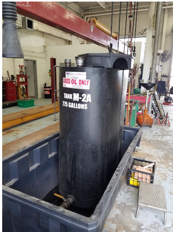
275-Gallon Tank for Used Oil (M-2A) Inside Maintenance Shop (Building 9)
