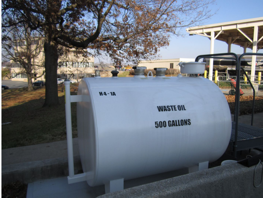
500-Gallon Used Oil Tank (H4-1A) At Hangar 4
