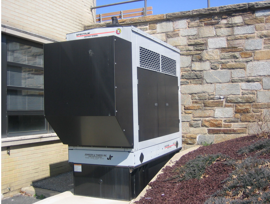
135-Gallon Diesel Fuel Emergency Generator Sub-Base Tank (ADM-1A) Outside Terminal Building
