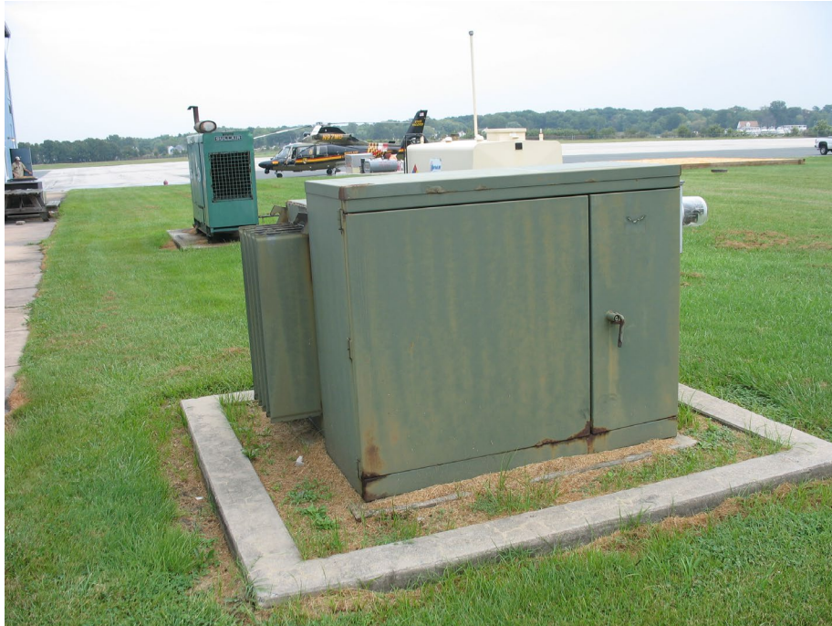
Transformer East of Maryland State Police Facility (Building 13) (MSP-1T)
