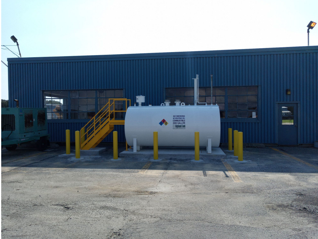
2,000-Gallon AST for Heating Oil (M-3A) Outside Maintenance Shop (Building 9)
