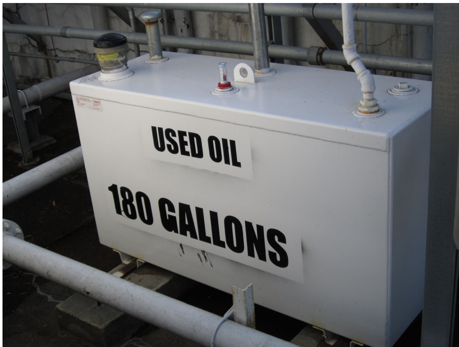
180-Gallon Used Oil Tank (FF-4A) At Fuel Farm – East Containment Area
