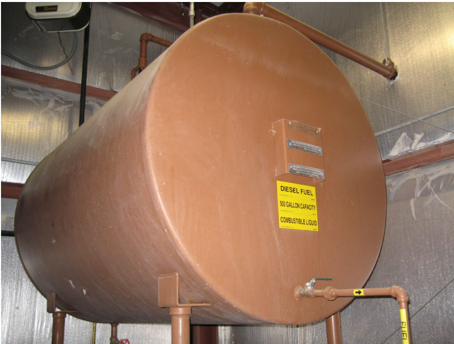
One of Three 500-Gallon Diesel Fuel Supply Tanks (FPH-1A through FPH-3A) To Fire Pumps Inside Fire Pump House
