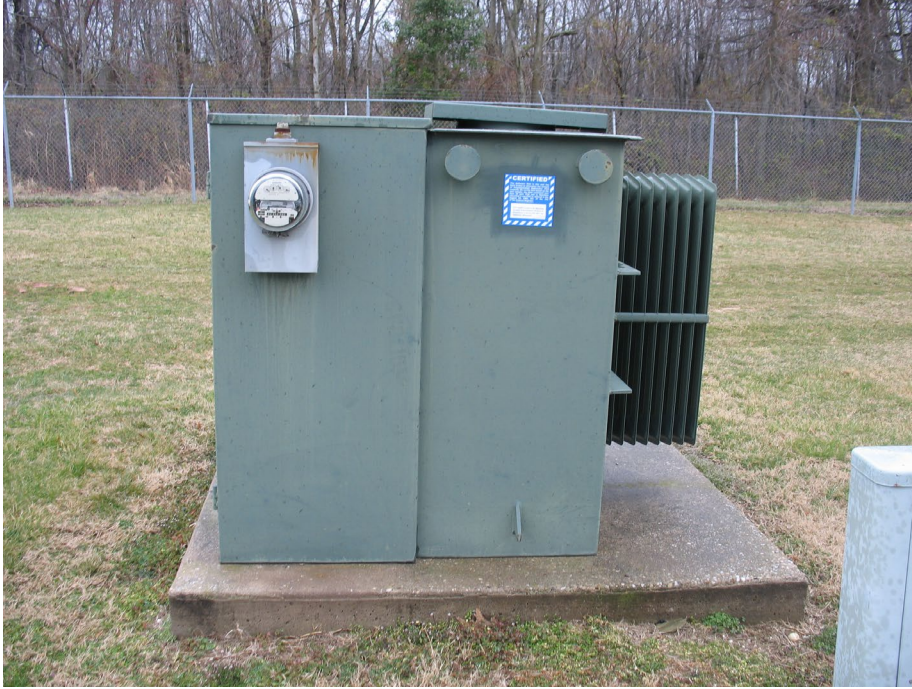
Transformer West of Maryland State Police Facility (Building 13) (MSP-2T)
