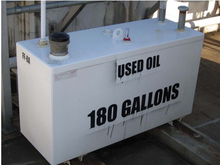
180-Gallon Used Oil Tank (FF-8A) At Fuel Farm – East Containment Area
