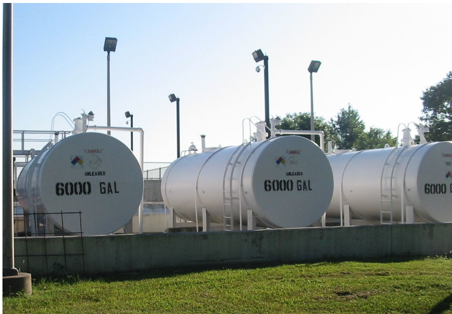
6,000-Gallon Unleaded Gasoline (FF-9A and FF-10A) and Diesel (FF-11A) Tanks At Fuel Farm – South Containment Area
