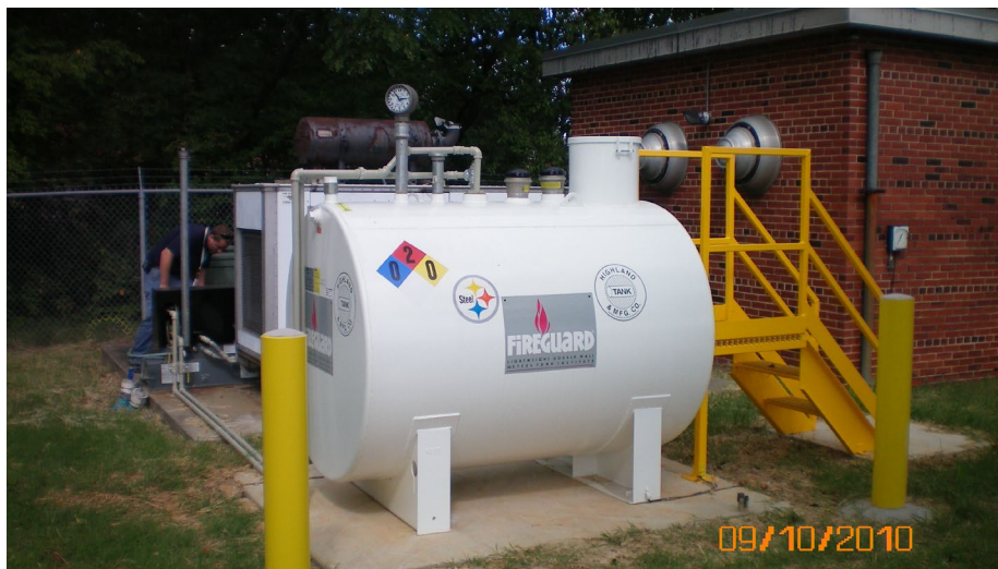
500-Gallon Diesel Fuel Supply Tank (RS-1A) to Emergency Generator At Field Lighting Vault
